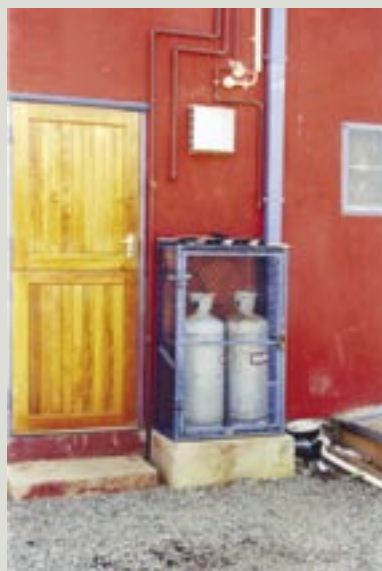
All units are fitted with gas for heating and cooking
