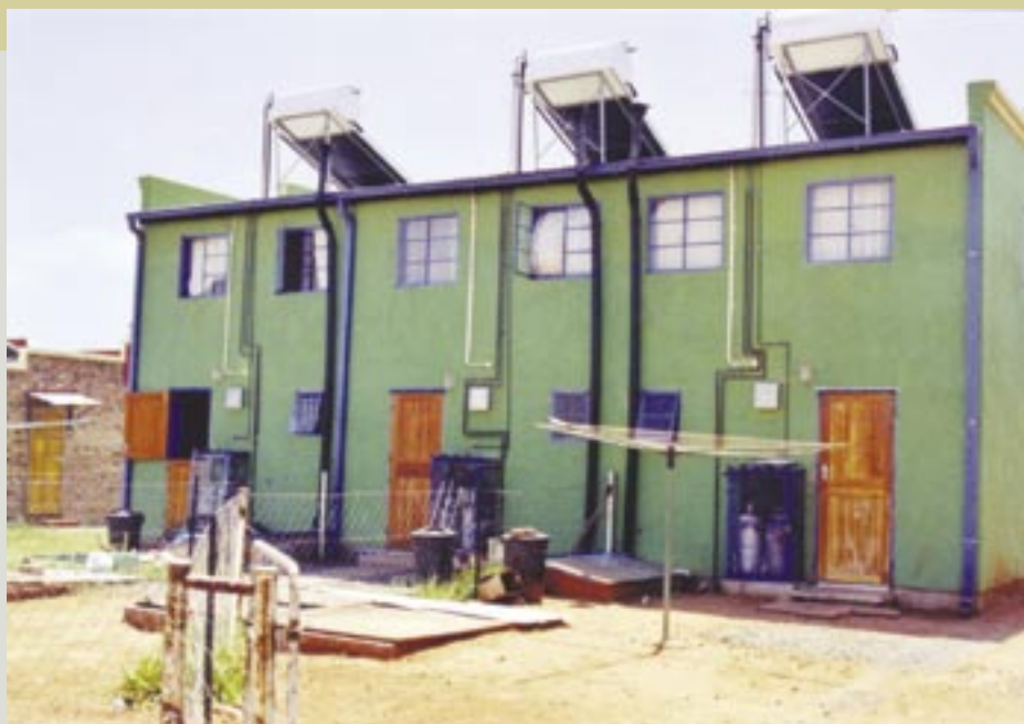
Solar water geysers are situated on the roof of each unit
