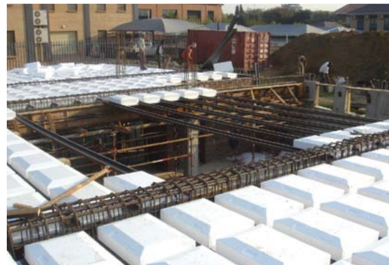
The TASS system from Automa Building Products is now being taken to the market by the supplier, Automa Building Products. To date over 50 000m 2 of TASS slabs have been successfully installed in the Gauteng area.
